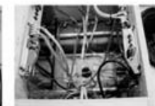
Internal amps and wiring
